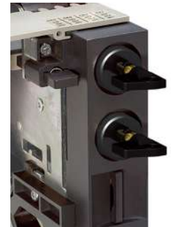
"Disconnected" position locking by keylocks.
